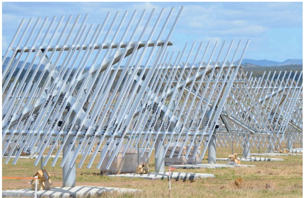
The solar photovoltaic research facility under construction on the UQ Gatton Campus.
